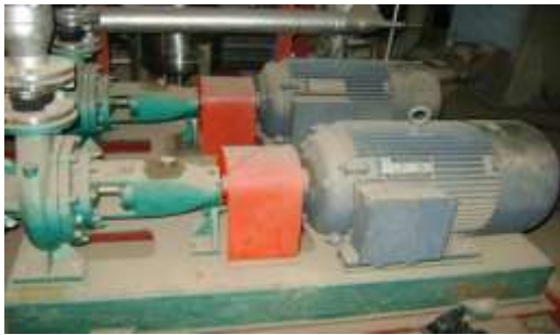
Gambar 3. Foto Generator Stator Cooling Water Pump 2B
