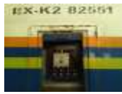
Gambar 2.1 Junction Box K2
