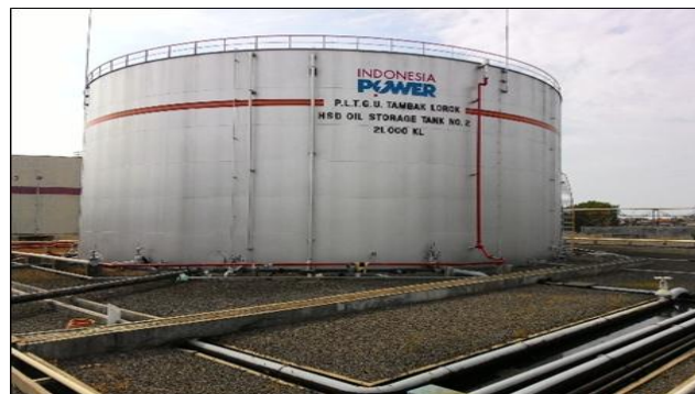
Gambar 1. HSD Oil Storage Tank
